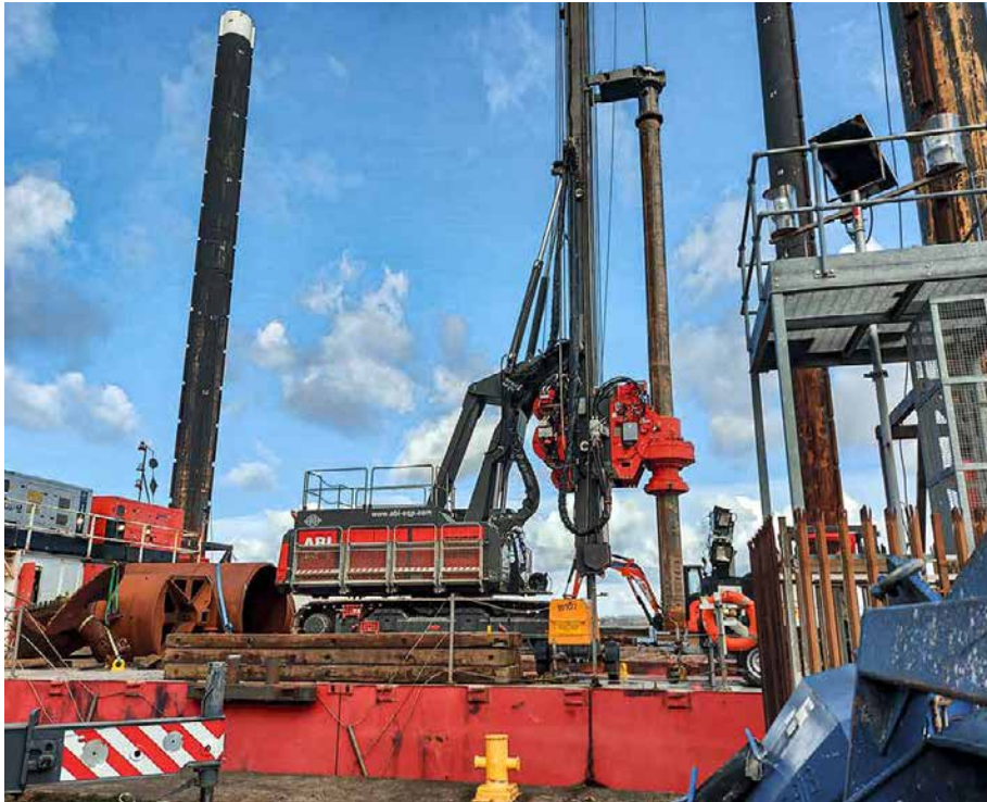
Photo: DELMAG drill rig RH 34 with Kelly bar guiding on a jack-up barge in port of Liverpool
