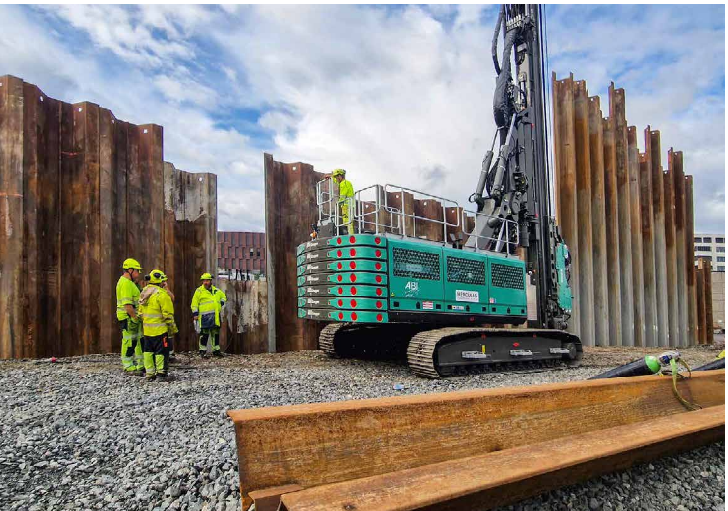
Photo: ABI MOBILRAM TM 20 with vibrator MRZV 30VV on the job site in Drammen
