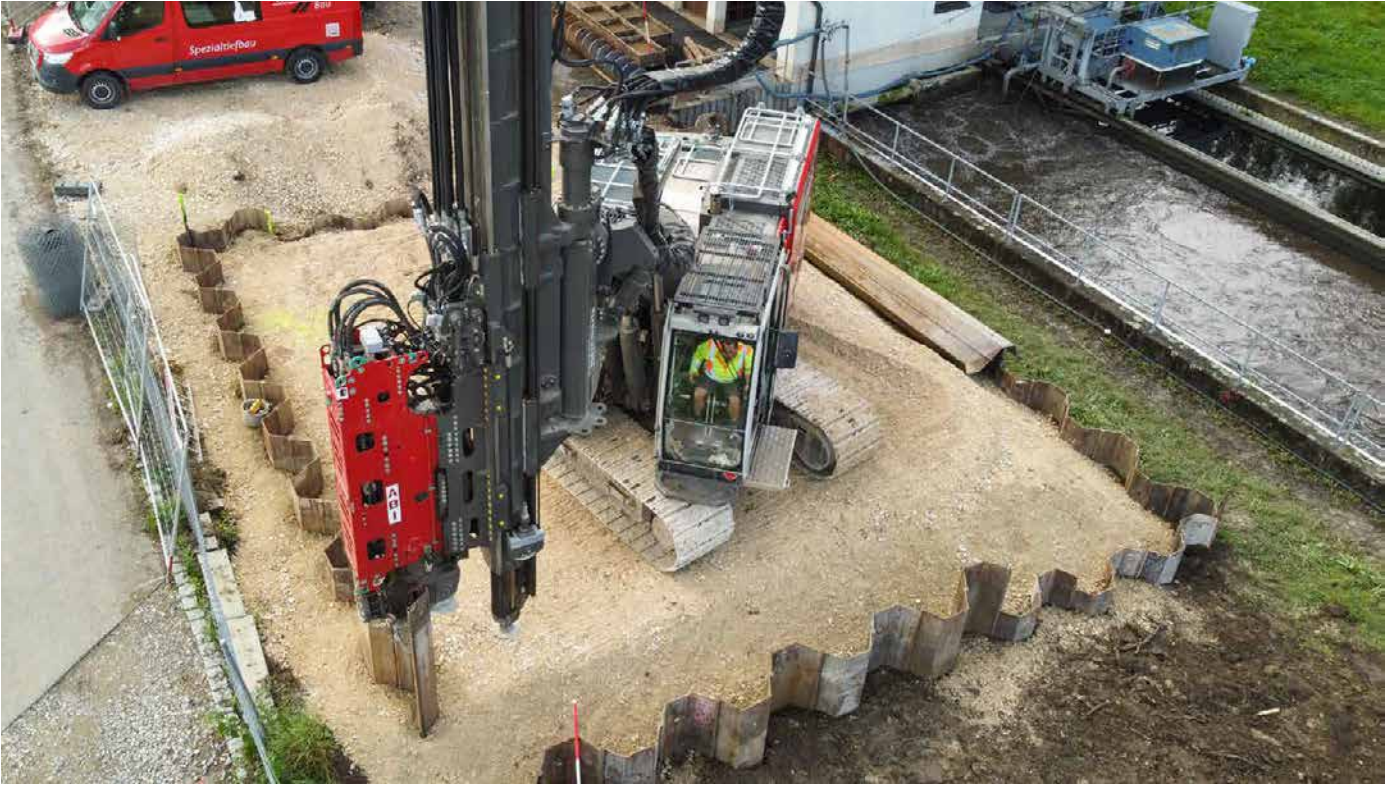
Photos: ABI MOBILRAM TM 14/17 SL while working at the job site in Inzigkofen-Vilsingen (above) Loading the machine for the transport to the next job site (below)
