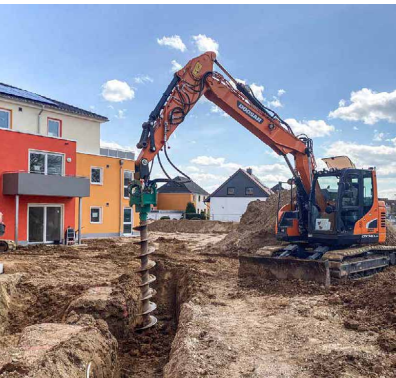
Photo: uncased drilling for a geothermal probe with the ABI excavator mounted auger drive BA 2200
