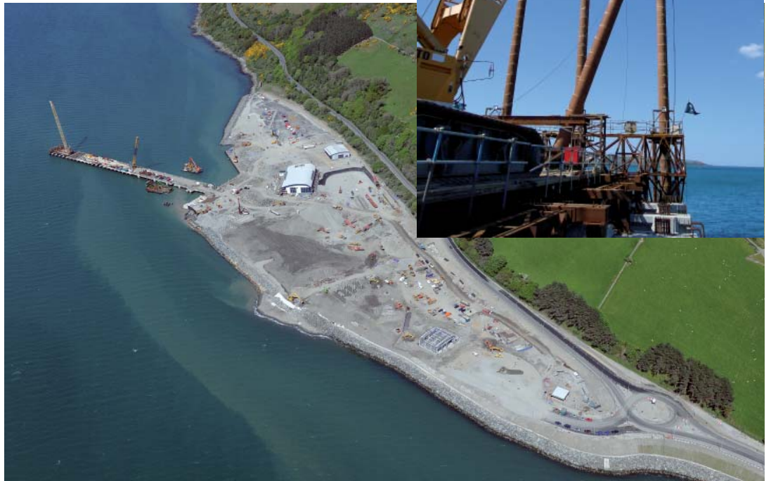
Photo: Aerial image of the job site at Loch Ryan, Detail: DELMAG diesel pile hammer D62 driving raked piles
