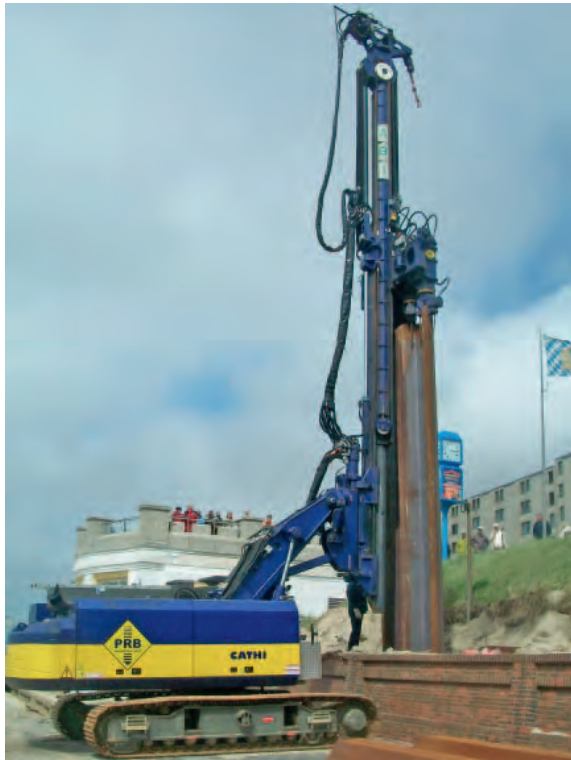
Static pressing with Hydro-Press-System: four steel sheet piles are pressed in a step sequence.
