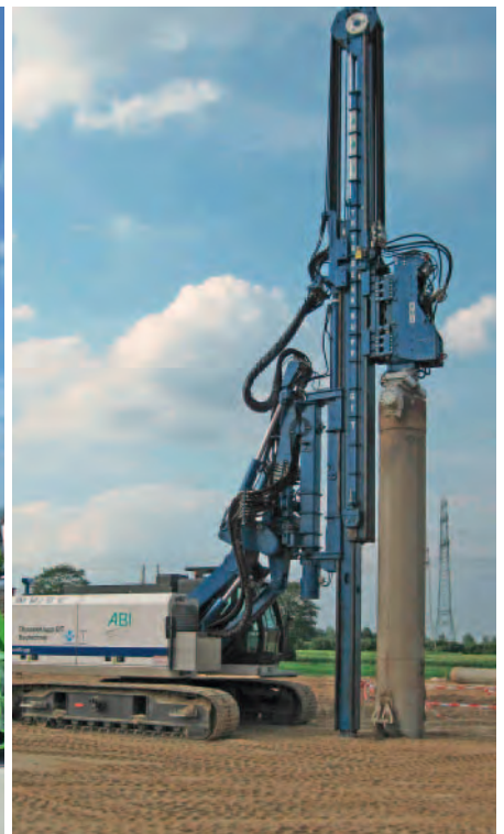
Installing geotextil piles: as a pile element a casing with reusable tip is used, after reaching the desired depth a fabric tube is inserted and filled with material.
