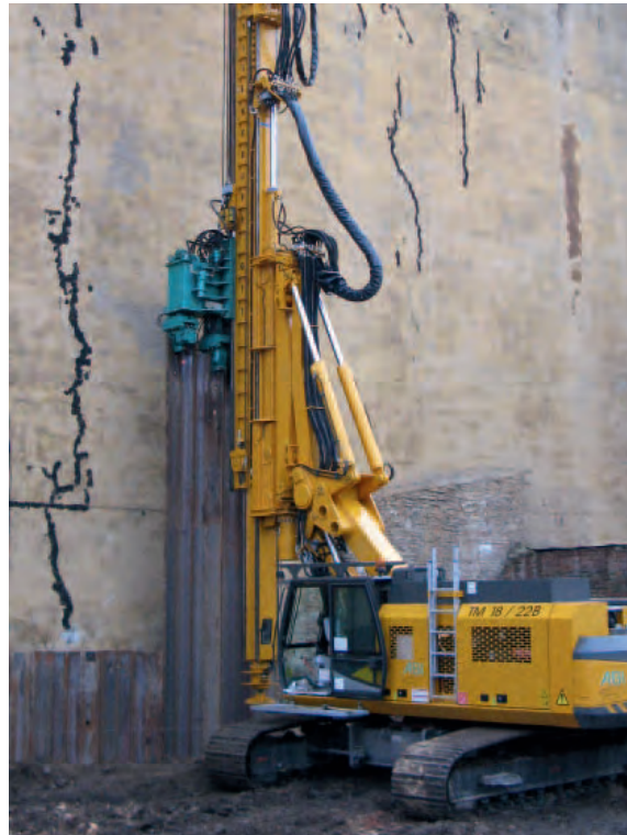
Static pressing direct in front of an existing building. In some cases the soil have to be loosened by pre-drilling before pressing.
