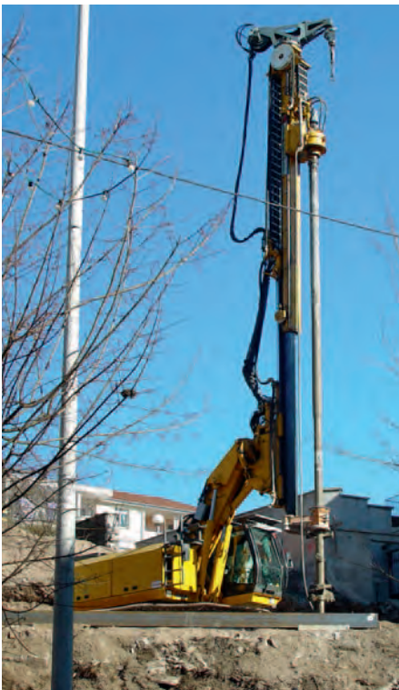
Soilmixing WSM: homogenous concrete piles are formed by mixing the existing soil with suspension while drilling and extracting the mixing tool.
