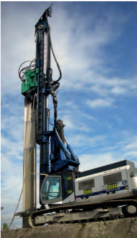
Installation of thin diaphragm wall as a sealing wall using a special H-beam. Displaced soil in form of the H-beam is filled with suspension.
