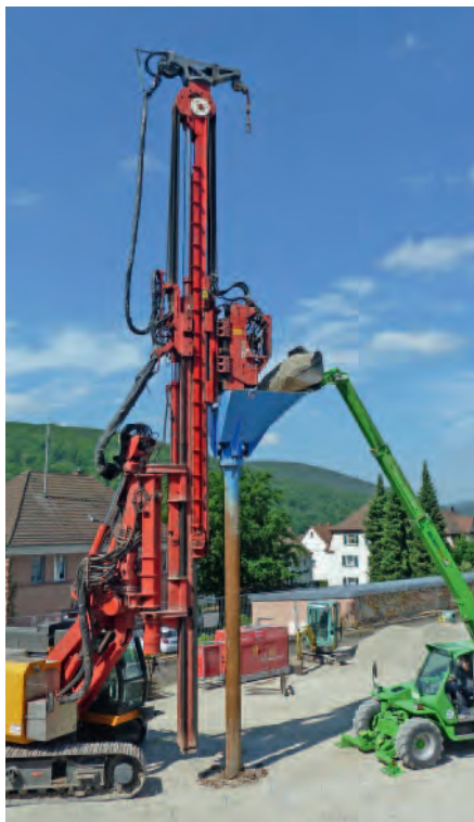
Stone columns: probe is driven to desired depth and while extracting the hollow space is filled and compacted with gravel using the pilger process.
