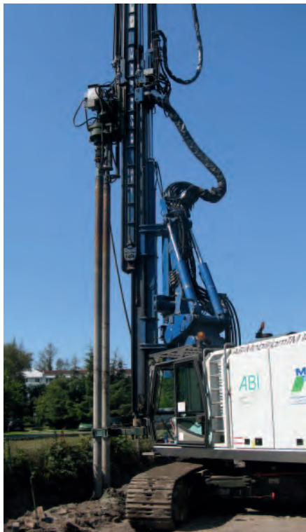
To achieve more efficiency the soilmixing procedure can be carried out as twin- or triplemix version, mixing two or three piles simultaneously.
