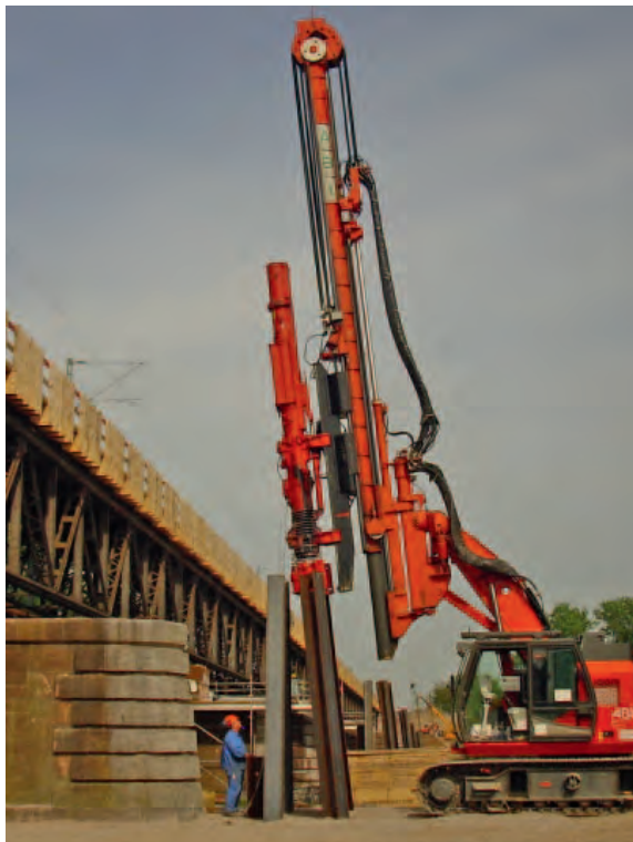
Impacting H-beams with DELMAG diesel pile hammer. With the DELMAG formula the load bearing capacity of the soil can be proved.
