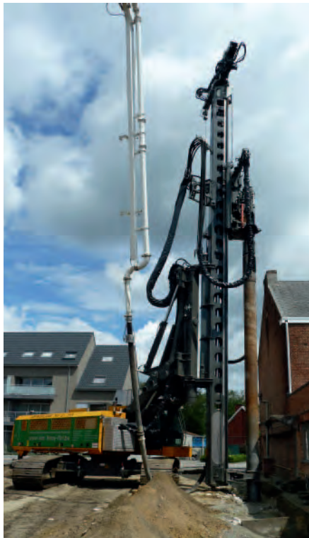
VDW drilling: the classic case of use - installing secant pile wall directly in front of existing structure.
