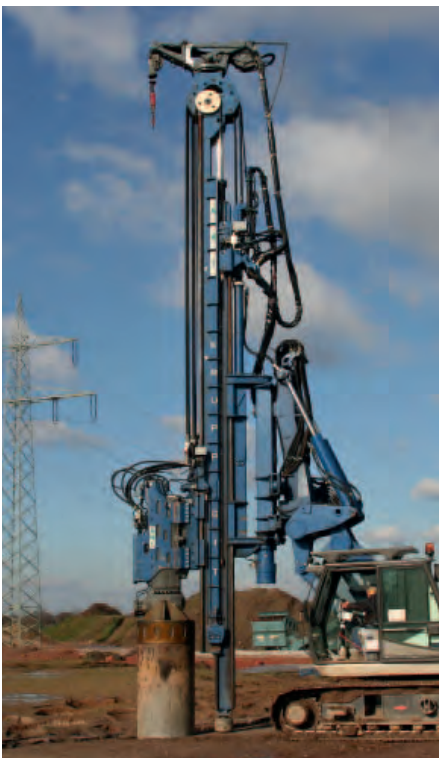
Soil improvement measure: large diameter casing is driven into the ground the resulting hollow space is filled with additional material.
