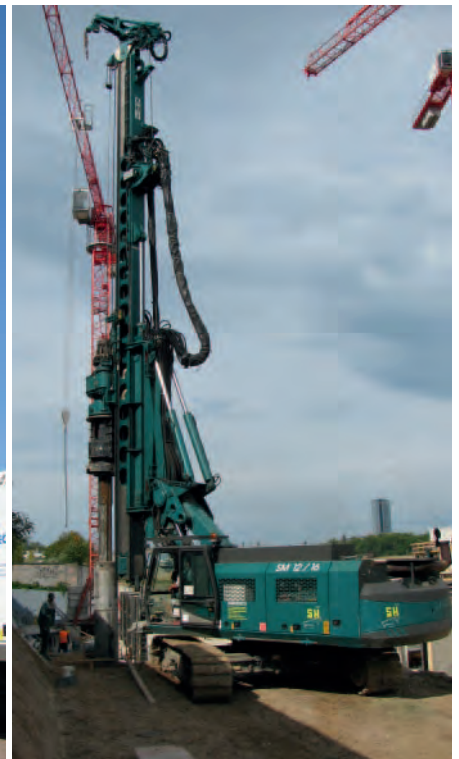
Kelly drilling: the machine is equipped with a kelly winch. The casing is drilled as deep as possible first and then drilled out with the auger. This process is being repeated till the requested depth is achieved.
